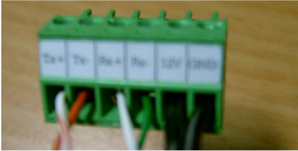
RS-422 Cable Connect to terminal block
